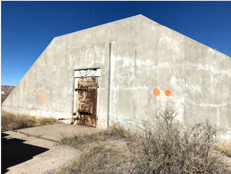
Photograph No. 2 Igloo A-947 Spray paint markings indicate where excavation is required
